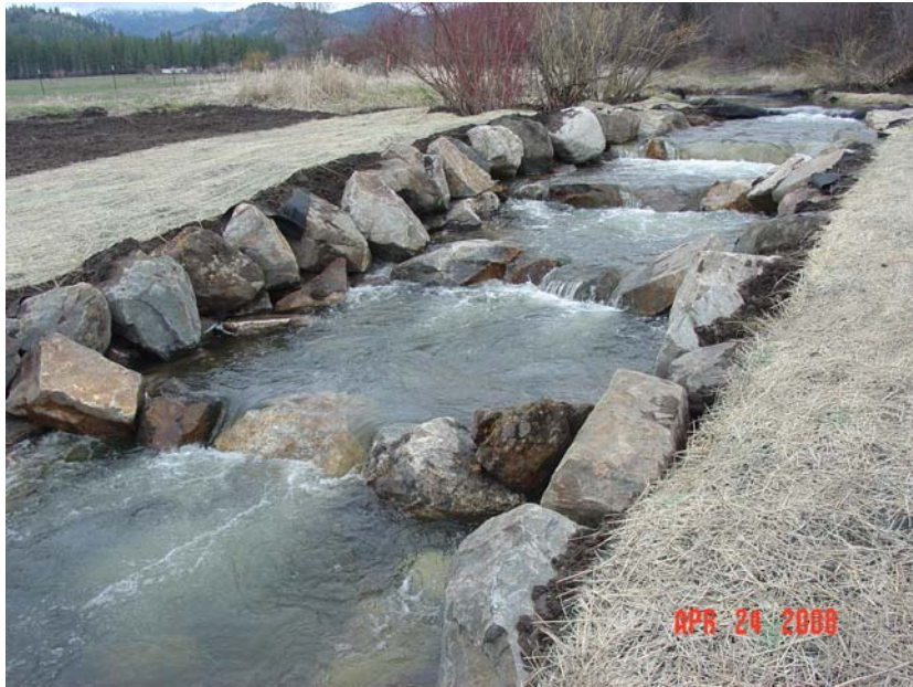
Figure 5. Photo depicting rock alignment and creation of pools. Erosion control blanket lines the bank.
